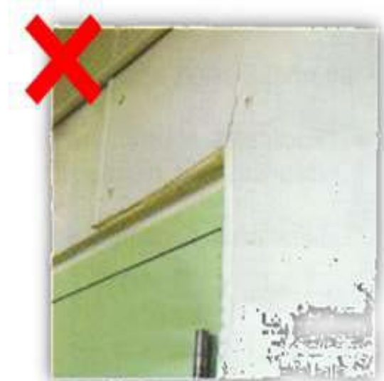
Cracks allow bacteria and molds to accumulate
